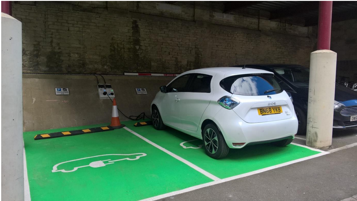
EV Charge point in use at County Hall. We have upgraded 3 out of our 7 pool cars to EVs and plan upgrade more by the end of 2019.
