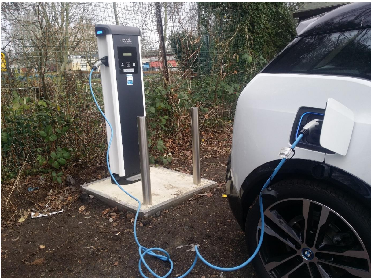
EV Charge point in use at County Hall.
