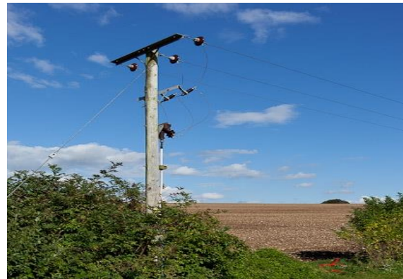
Lack of grid capacity
